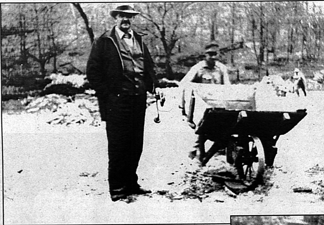
Whis Dye and Cliff Hammock (the grandfather of current Waynesville Mayor Cliff Hammock) are captured on film while working on the construction of the Old Hanna Store in the Late 1920's.
