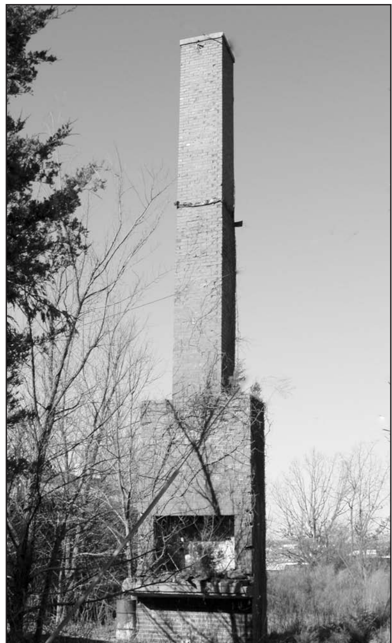
Only the chimney is left of the Colored USO Club on Missouri Avenue, just outside the main gate. Photo by Terry Primas.
