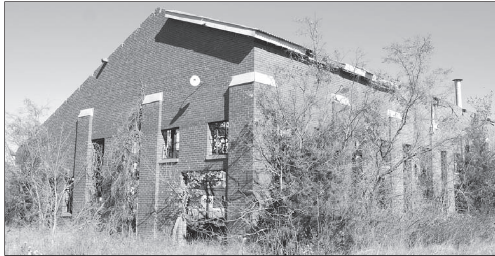
The main engine building of the Gulf Oil pump station still stands. Most of the roof of the sturdy brick and steel building is missing and the two huge diesel engines are long gone.
